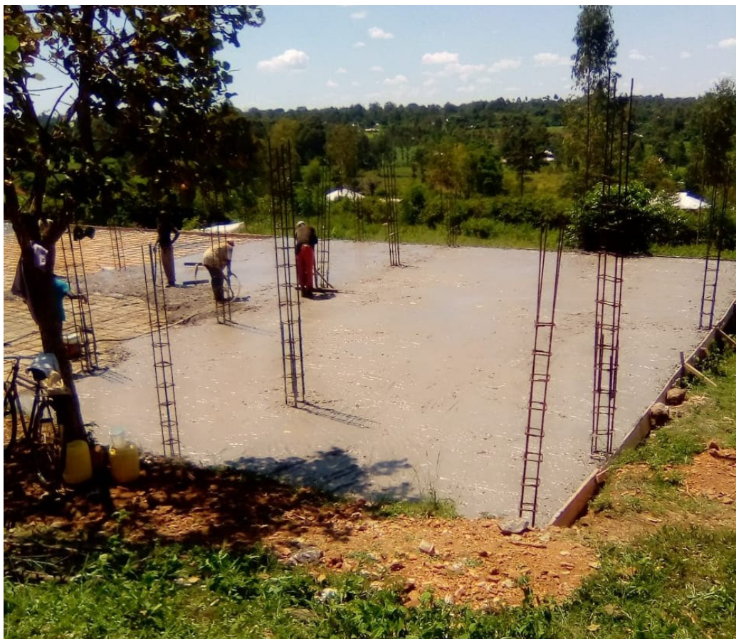
Foundation floor being laid for the ground floor of the new three storey building housing a dining area, teaching areas and dormitories.
